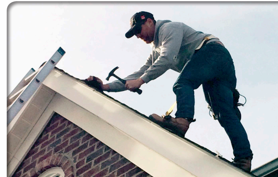
Heights are no match for David Silverstein, VP of Business Development, shown here installing a new roof for a customer.
